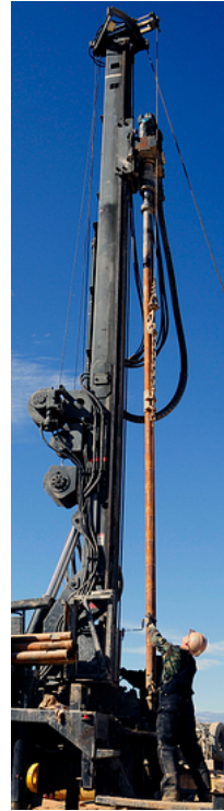
“US Navy 090226-N-9584H-018 Construction Electrician Constructionman Greg Langdon, assigned to Naval Mobile Construction Battalion (NMCB) 1, installs a new section of drill steel during a water well drilling operation” by Mass Communication Specialist Seaman Ernesto Hernandez Fonte via Wikipedia . Public Domain.
